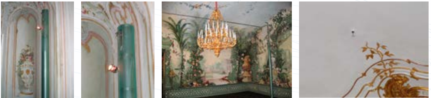
These images, taken in Schönbrunn Palace, are of a fire protection Totem, containing a suppression system, emergency lighting, public address system and a fire alarm sounder together with a sprinkler head in a decorative ceiling. Would you consider them a blight on the space? (Images courtesy of Schönbrunn Palace)
