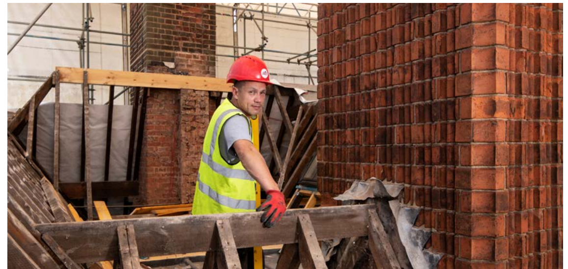
Carpenter working on roof structure beside fluted brick chimney, Highbury Hall, Moseley, Birmingham
