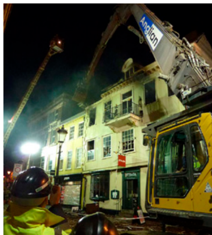
Cupola House, Bury St. Edmunds, first taken off the Heritage At Risk Register in 2003, has been put back on after a devastating fire. © English Heritage
