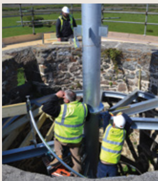
Image: The new spiral stair being installed at Landewednack Windmill, May 2015 (Historic England ©)
