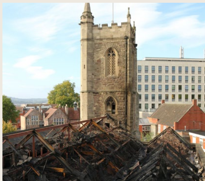
Image: Damage to the roof of St Michael on the Mount, Bristol following a major fire in October. © Avon Fire & Rescue Service.
