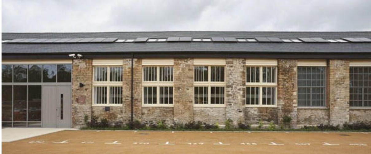
The Chain Testing House– before and after the renovation work. © Thomas Homes
