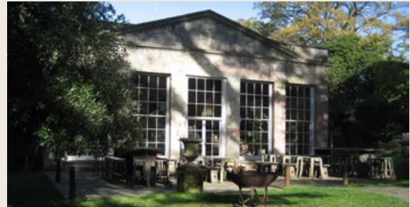
The Orangery at Combe House, Gittisham, East Devon, sensitively repaired and back in economic use. © John Clark
