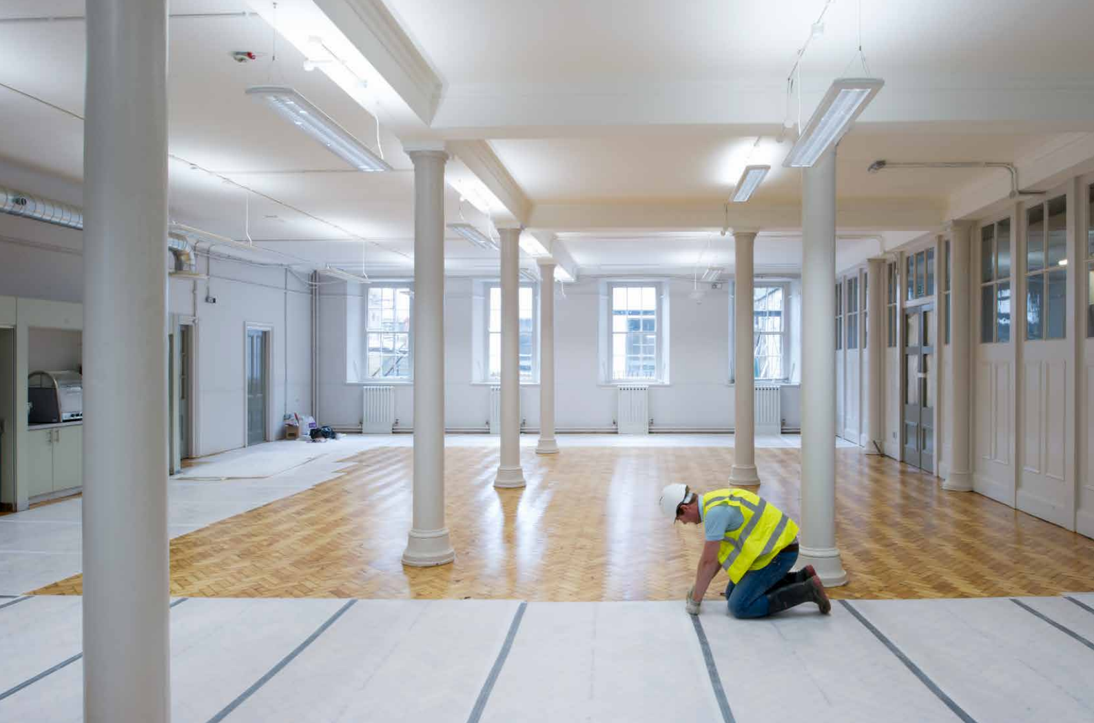
King Edward VII School Upper Site, Sheffield. First floor corridor showing old and new build together. © Historic England Archive
