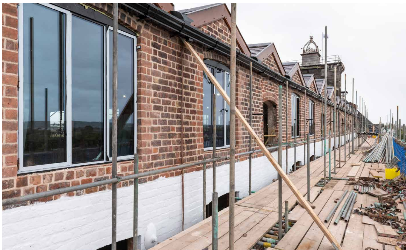
Metal window frames being installed at Shrewsbury Flaxmill Maltings, Shropshire. © Historic England Archive
