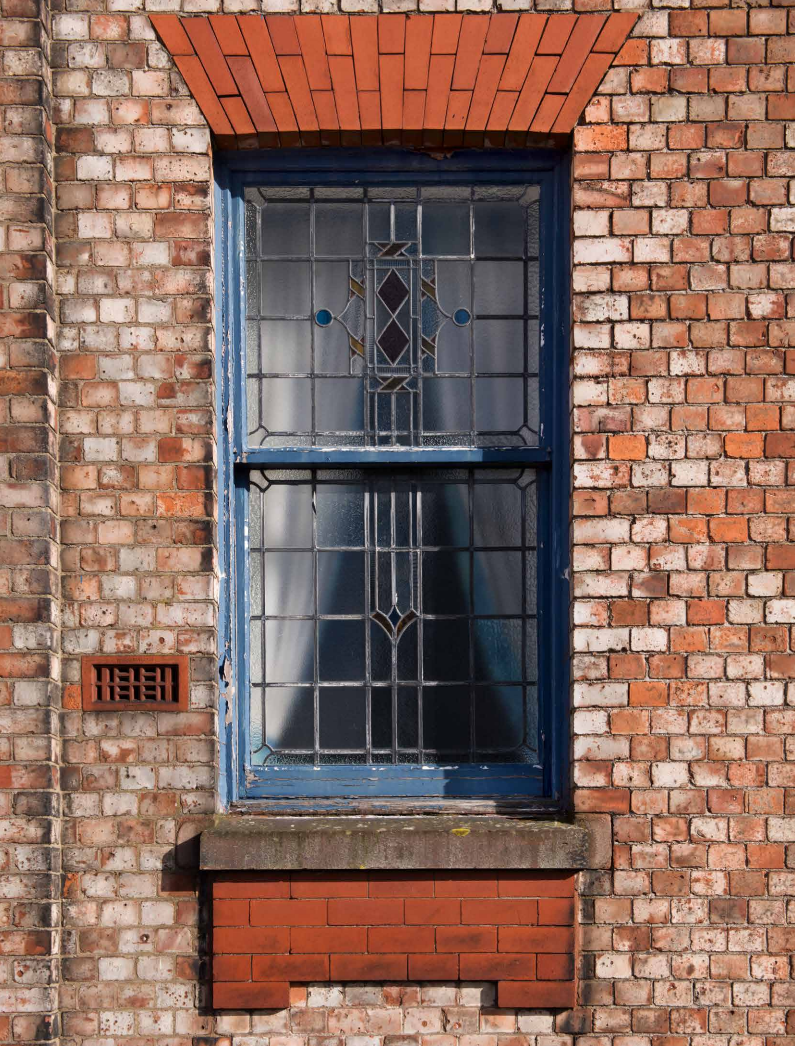
Traditional timber windows can have long service lives if well-maintained.. © Historic England Archive
