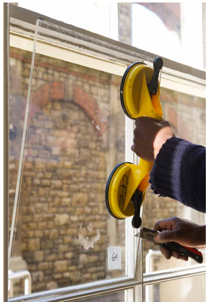
Right: Installation of secondary glazing at The Engine House, Swindon, Wiltshire. © Historic England Archive
