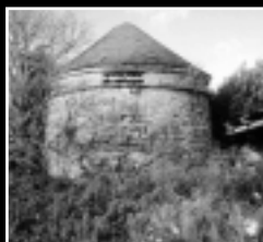
A dovecote at Barnby in the Willows, Nottinghamshire. This is a rural building in decline and a Building at Risk.
