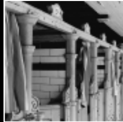
Changing facilities await restoration
