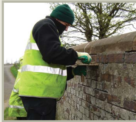
Image Craftsmen working on the Birmingham & Fazeley canal. Traditional craft skills are highlighted in Putting the Historic Environment to Work .
