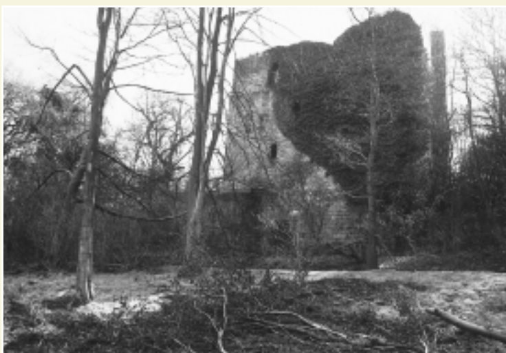
HAREWOOD CASTLE A view of the ruins of Harewood Castle from the north-west. As part of the agreed programme of repairs, the collapsing arch on the Castle's south-west elevation will be consolidated and loose masonry to the wall-tops reset. The setting of this monument will be restored through the removal of inappropriate tree planting.
