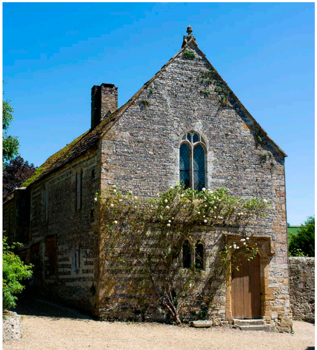
Figure 12: Guesthouse, Cerne Abbey. Cypris Freestone and flint, Ham Hill Stone, and Portland Stone.
