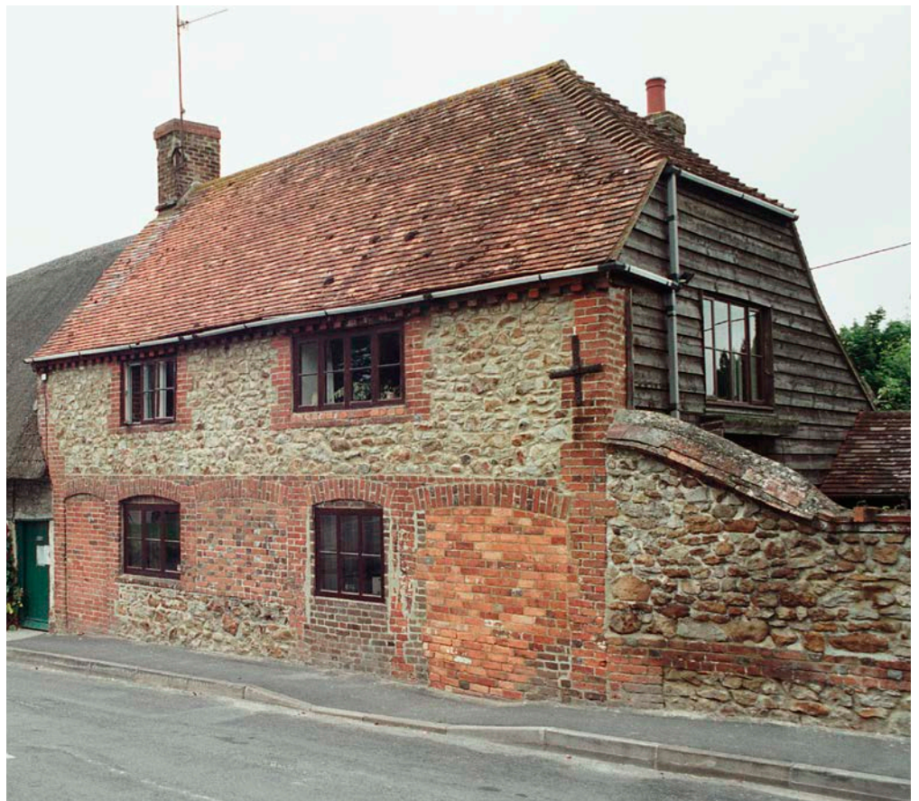
Figure 15: Old Forge Cottage, High Street, Ashbury, Vale of White Horse. Uncoursed Sarsen Stone rubble with brick quoins and dressings.
