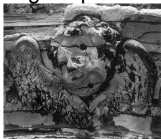
Detail of plaster modelling showing typical problems of broken edges, soft undercoat and splitting from iron nails.
