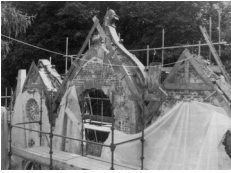
Repairs tinder way to the 'Museum' building at Enville, Staffs, one of a number of mid eighteenth century garden structures recorded before extensive repair
