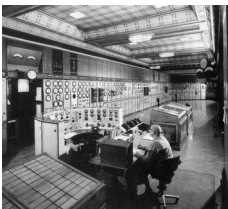
Battersea Power Station, the Control Room in use (CEGB)
