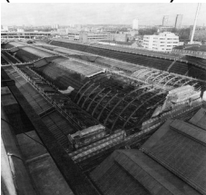
Paddington station roof seen from above, showing the work in progress on the first stage (British Rail)
