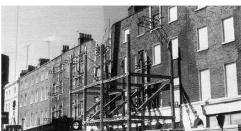
Front elevation of Manchester Street following second collapse, May 1990 (Westminster City Council)
