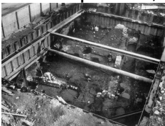
Excavations at the Stakis Hotel site, Wellington Row, York, revealing the remains of a Roman warehouse of second century AD date
