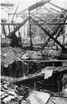
View of the Grace and Favour apartments the morning after the fire (PSA)
