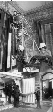
The removal of curtains in the Morning Room ready for treatment (above) and loading the wrapped textiles into the deep freeze (below)
