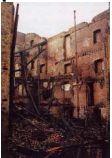
Tall, unrestrained walls and weight of fallen debris are problems here (note freestanding cast-iron column)
