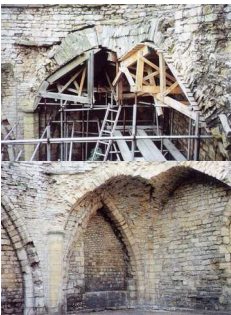
The kitchen, Bishops Palace, Lincoln: the vault at the northwest corner before and after consolidation
