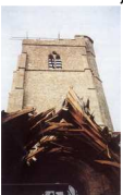
Collapse of the spire in a storm threatened the stability of the nave
