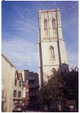
Bristol Temple church: typical church tower that has been leaning for many years
