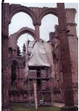
Experimental treatment with Brethane alkoxysilane at Goodrich Castle, a project started in the mid 1970s
