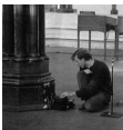
Figure 3 Monitoring of tile pavements at Westminster Chapter House; Dr Timothy Yates, BRE
