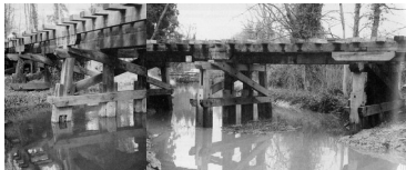
Wickham Bishops Timber Trestle Railway Viaduct, Essex. A unique survivor – though now disused – of a once common viaduct. Essex County Council, grant-aided by English Heritage, restored it.
