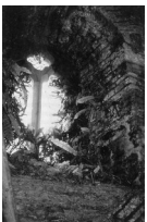
The ferns growing inside the reveals of the west window in the tower before the cementitious mortar was removed from the outside
