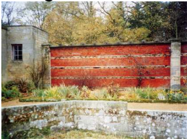
South face of hot wall before repair
