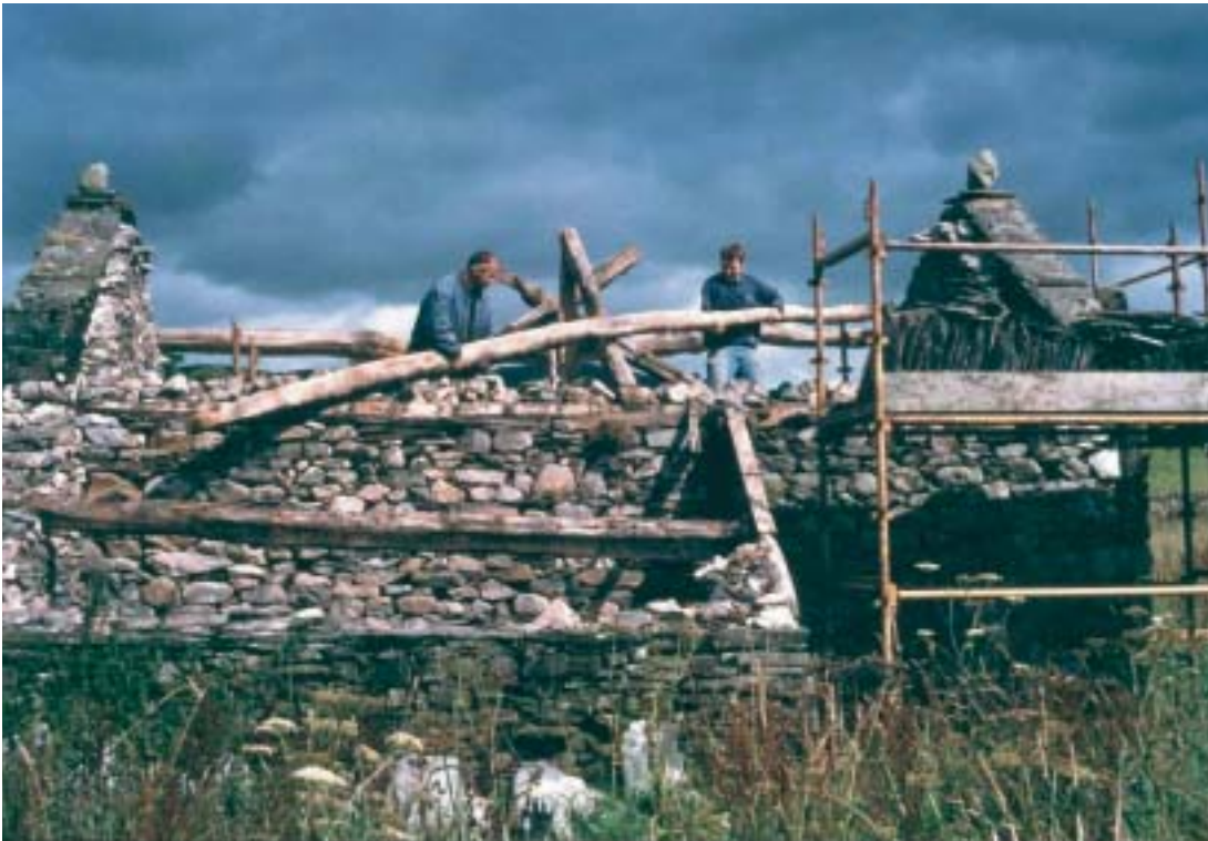
Agri-environment schemes have rescued many farm buildings, particularly within our visually most striking landscapes. Here, Ecclerigg Barn is repaired as part of the Lake District Environmentally Sensitive Area scheme
