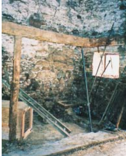
Penruddock, Cumbria, Grade II. The rotten floor in this byre was removed at the request of DEFRA
