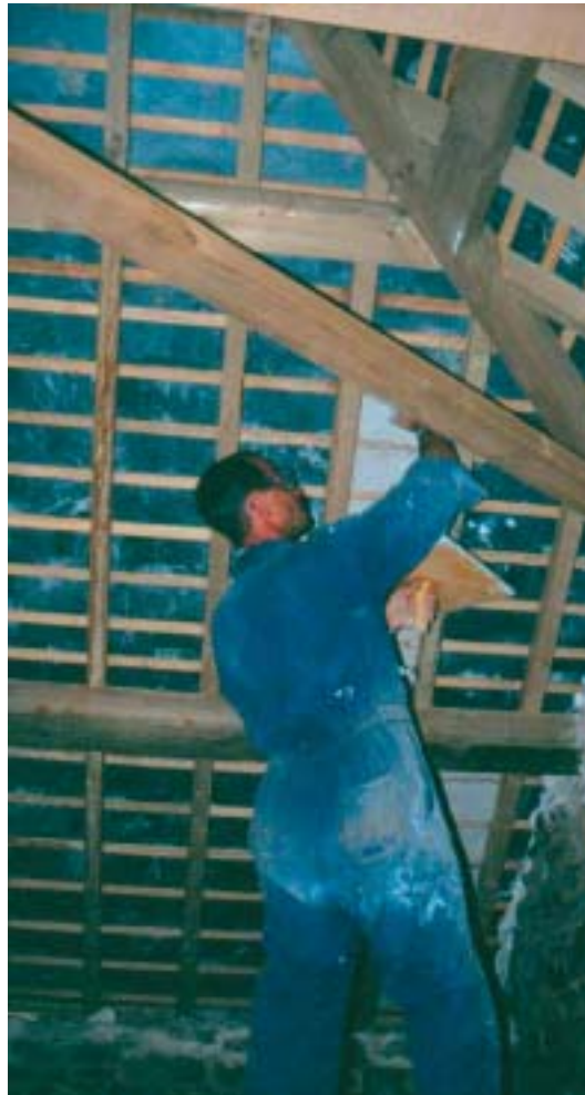
Local craftsman 'torching' (applying lime plaster to the underside of the slates) the roof of a farm building, as part of a project funded through the Dartmoor Environmentally Sensitive Area scheme. Rural Development Programme projects conserve the historic environment, help keep craft activities alive and create employment
