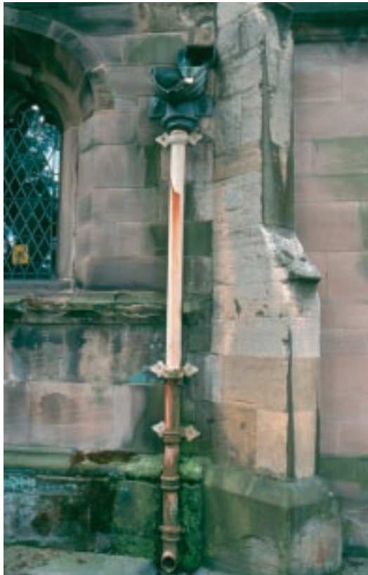
Blocked rainwater hopper and pipe in urgent need of maintenance
