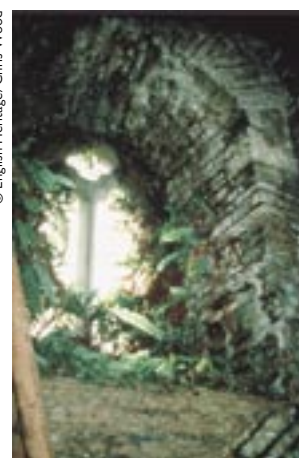
Callacombe Church, North Devon, showing the effect of driving rain constantly soaking the walls. The tower was repaired four years ago (see Conservation Bulletin 36, 14–16).
