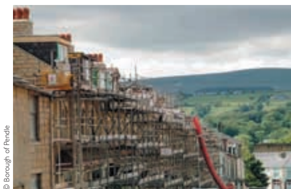
Nelson, Lancashire. View of Whitefield ward, showing housing repair work under way in the context of the wider landscape. Pendle Hill is visible in the distance.
