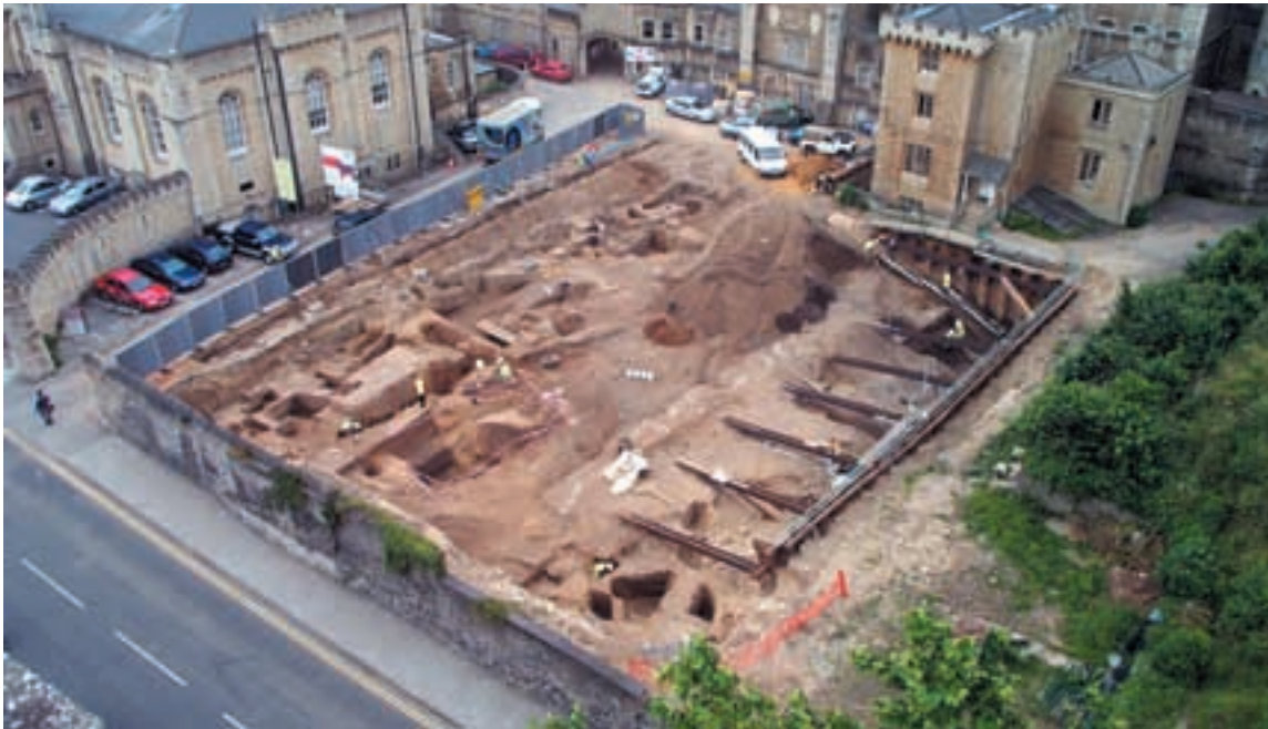
Professionals working together. Oxford Castle shows the full range of professional skills needed today for regeneration of the historic environment.
