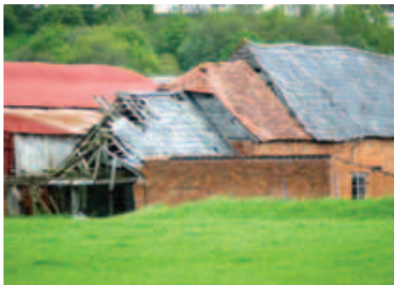
Redundant historic farm buildings may be an asset to the landscape, but their repair can be a significant drain on the resources of their owners.
