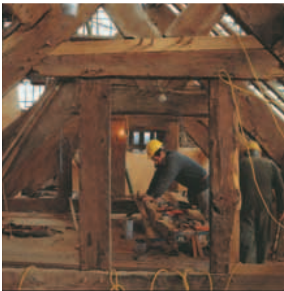
During the 1990s Cadw undertook a major programme of conservation on the Elizabethan town house of Plas Mawr in Conwy. Both the conservation and subsequent presentation were well informed by thorough research and understanding. © Cadw, Crown Copyright
