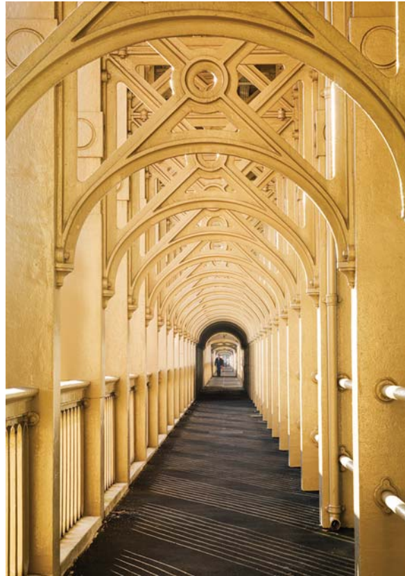
The High Level Bridge between Newcastle-upon-Tyne and Gateshead was designed and built by Robert Stephenson in 1845–9. Recently the subject of a major programme of repair it remains one of the glories of Tyneside and a masterpiece of infrastructure engineering. James O Davies © English Heritage
