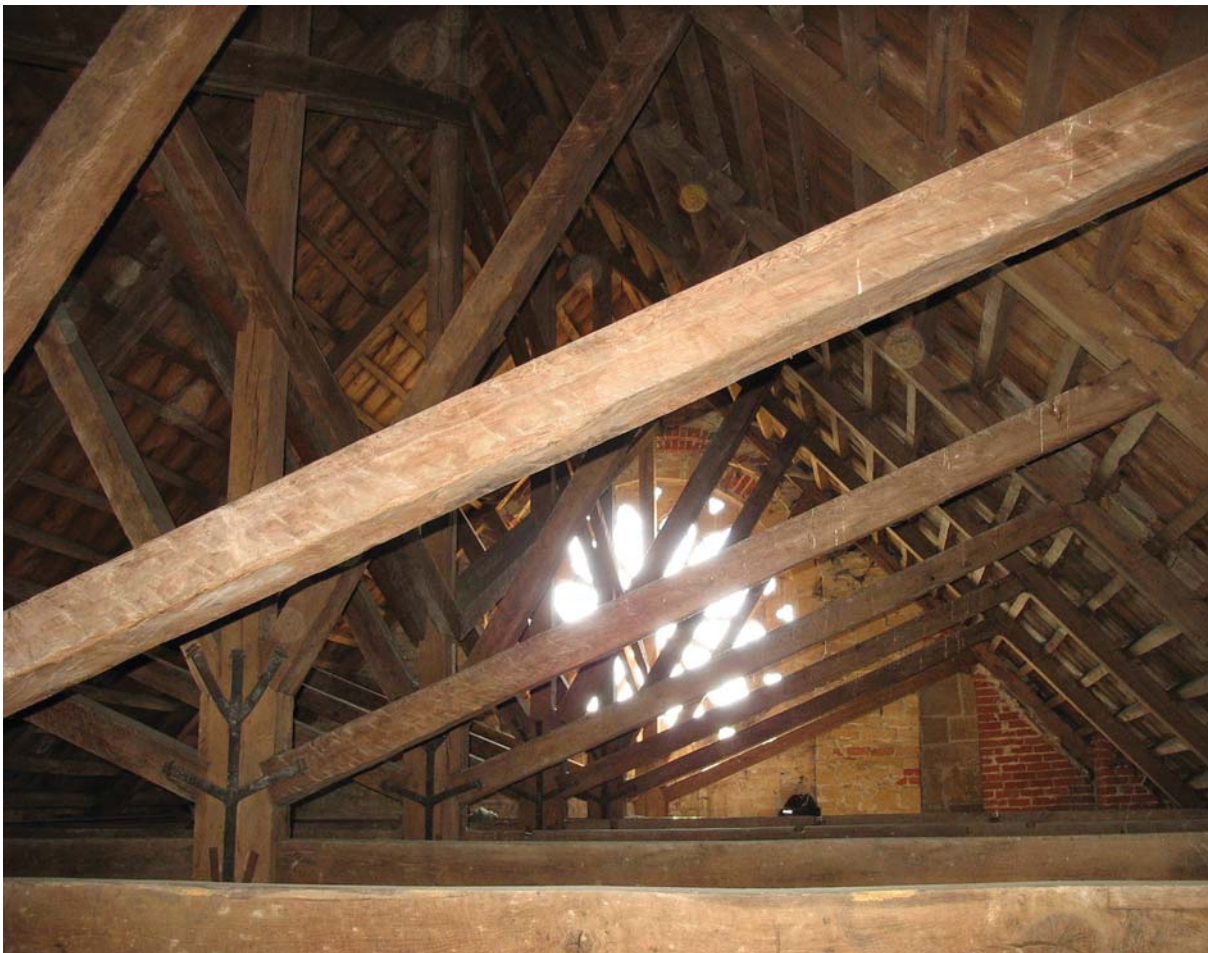
Slow-growing and thus durable Baltic pine was used for most of our historic buildings between 1750 and the end of the 19th century.
