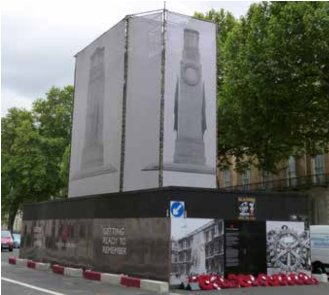
Image 95 Cleaning and repair work in hand on the Cenotaph, Whitehall during 2013. © Odgers Conservation Consultants.
