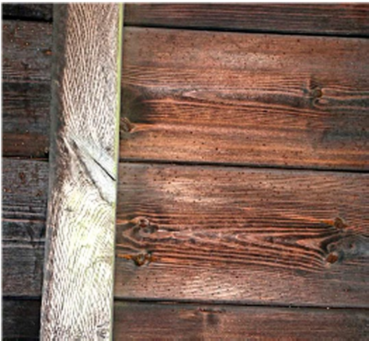
Figure 3.9: A common furniture beetle infestation can be seen in the cover boards on the underside of this lychgate roof. Damage is generally restricted to sapwood. Active beetle infestations usually only occur where the timber is damp.
