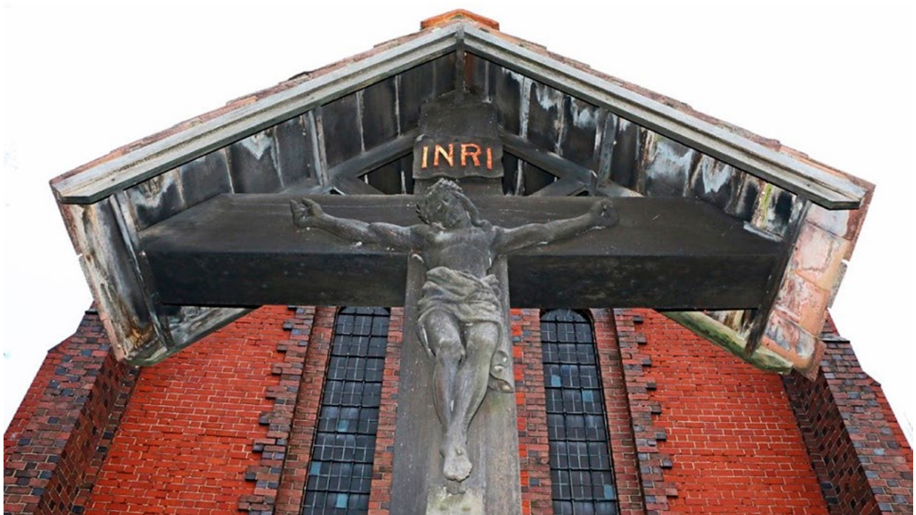
Figure 3.10: The underside of this Calvary roof shows staining and decay from water ingress caused by pointing failure below the edges of the tiles.
