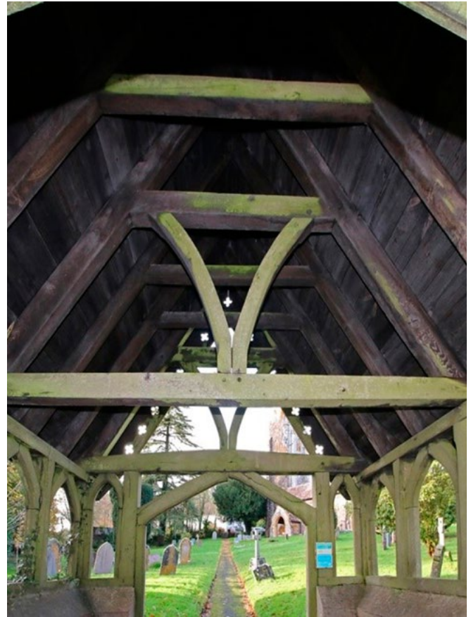
Figure 3.6: Algal growth on lychgate timbers indicates persistent dampness, the cause of which needs to be investigated.
