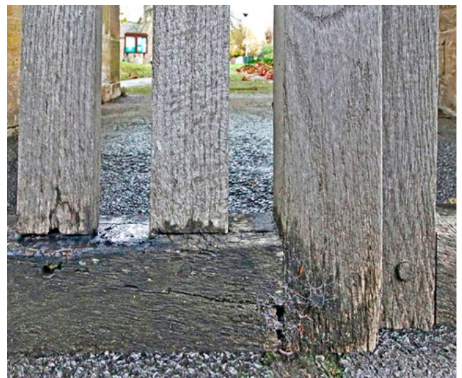
Figure 3.8: Decay in the bottom rail of this gate is the result of its exposure to the elements, as it is farthest away from the protection of the lychgate roof and within the 'splashback zone' from groundwater.
