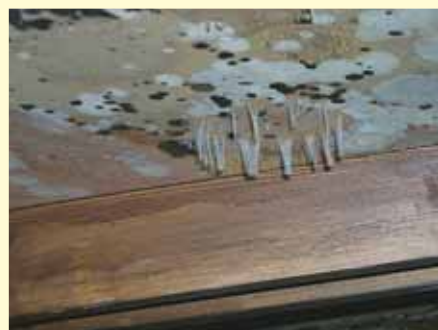
Fig 10 (above) Mould growth on telephone exchanges and under plotting table.
