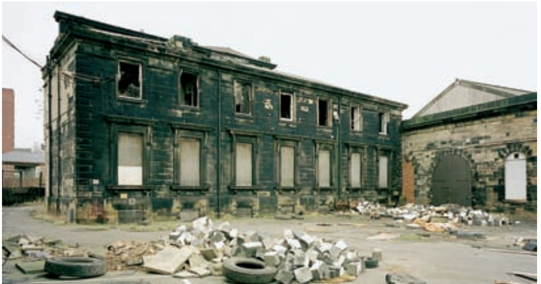
Fig 2 Former station hotel, 1844, at Greenesfield by G T Andrews of York; it was dismantled in 2003. The later engineering workshops can be seen on the right of this view. [AA028727]
