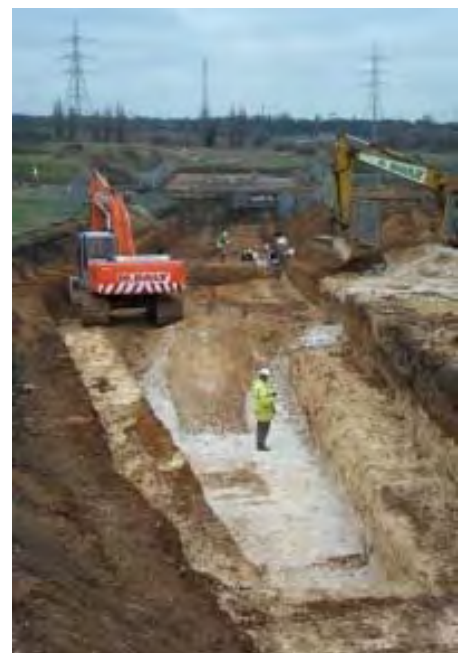
Fig. 6: Investigating the Palaeolithic during construction of Channel Tunnel Rail Link (Photo: Rail Link Engineering)
