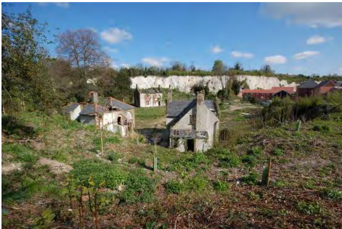
Fig. 31: Derelict historic buildings in Botany Pit (also known as Church Hollow) Purfleet. These are being recorded prior to renovation
