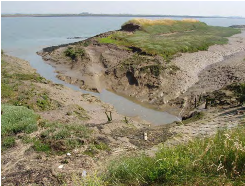
Fig. 19: Managed realignment at Wallasea; the cut through the seawall © Copyright David Williams and licensed for reuse under this Creative Commons Licence .
