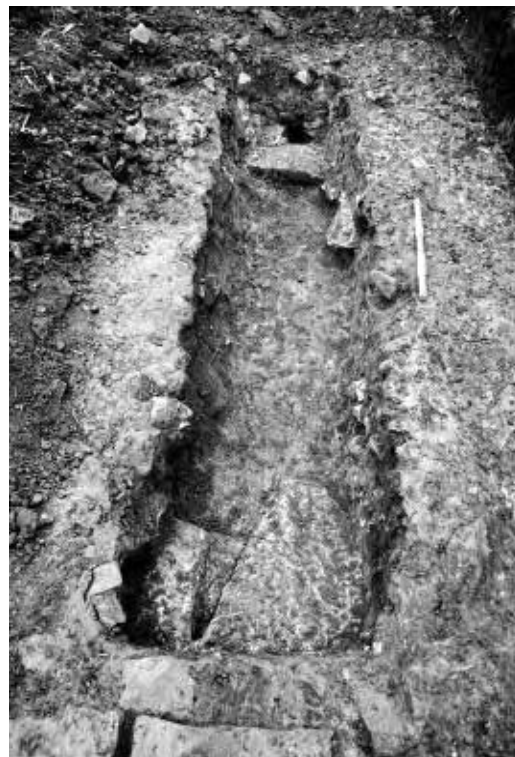
Fig 248 Milecastle 10: photo of Trench 1 showing section through robber trench and surviving wall face.
