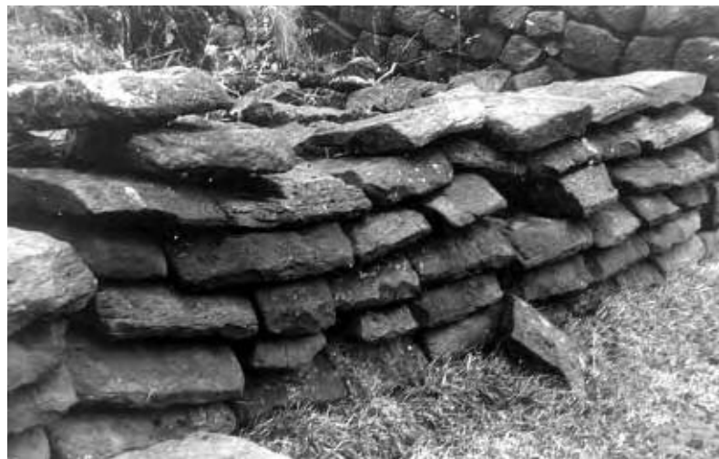
Fig 180 Consolidation on the north face of the Wall at Thorny Doors, where the original Wall face was 10ft (3.05m) high.
