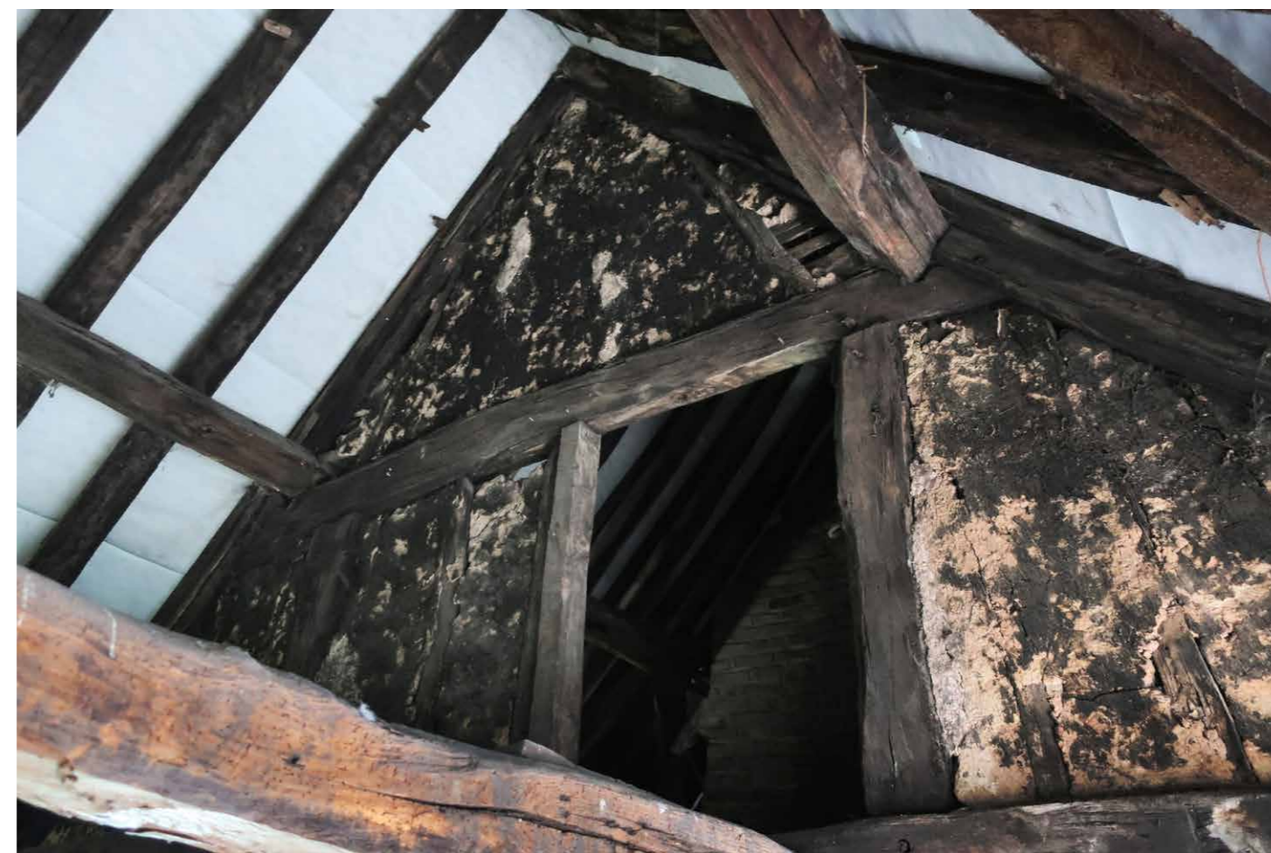
Above right: Soot from the fire still visible in the roof structure of the smoke bay in the detached kitchen range. © Historic England, IMG_6686
