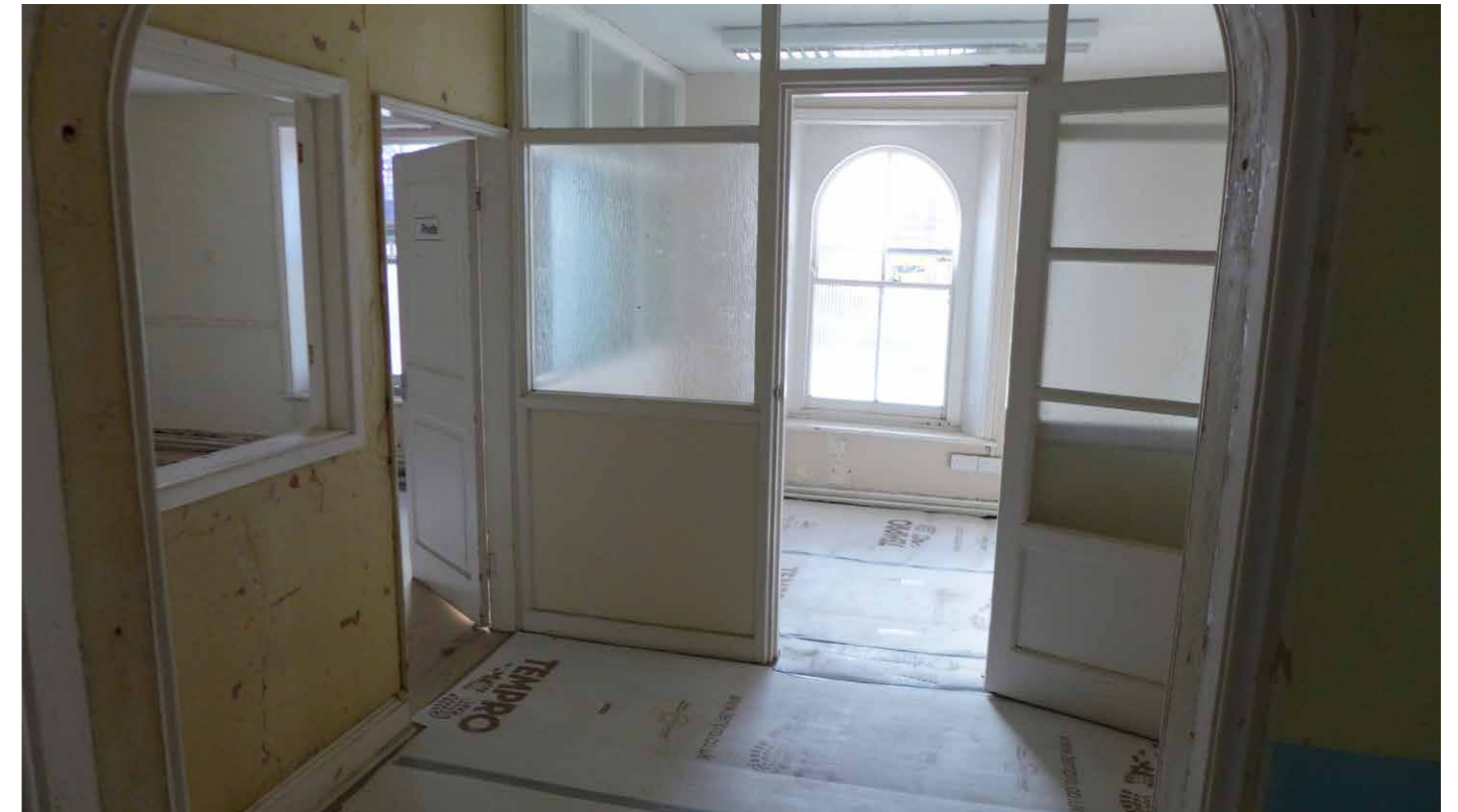
Above right: Conversion of The Cedars as council offices involved various changes, undertaken around the late 1950s/early 1960s. The post-war features in this image have recently been removed and the area opened up as part of the adjacent room. © Historic England
