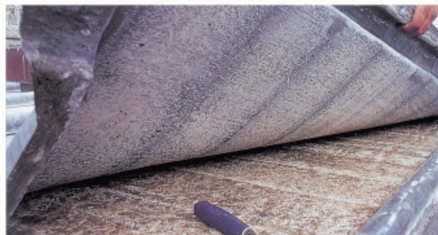
Figure 5 A quinquennial inspection found a compact layer of white corrosion product under this roof on a historic house in Dorset. Over most of the roof, lead which was wire-brushed clean did not corrode again. It was concluded that most of the corrosion had occurred during or shortly after re-roofing, when the lead was vulnerable and the substrate timbers were damp. Coatings of various kinds can help to protect fresh lead from this initial corrosion: see Section 6. At the bottom right, note also the mild corrosion originating from the distillation of rainwater trapped in the splashlap by capillary action. This is discussed further in Section 3.
