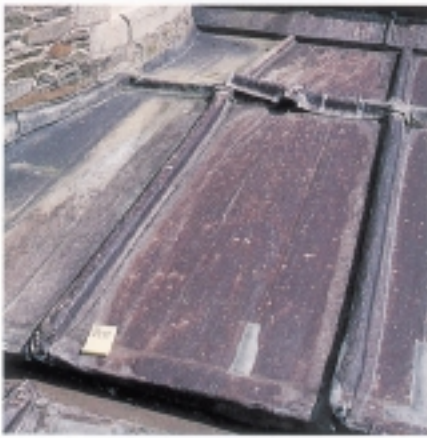
Figure 2 This 1850s roof has eventually failed owing to fatigue cracks caused by thermal stresses in large sheets subject to constant thermal movement. A small amount of ULC was also visible under the sheets: this is perfectly normal, and has not contributed significantly to the failure.
