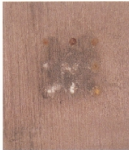
Figure 1 The corrosion behaviour of lead is markedly affected by small changes in environmental conditions. This test specimen, near actual size, was placed on a sheet of polythene-backed building paper on softwood and subjected to evaporation / condensation cycles for two weeks. The paper had nine pinholes in it: above these, dots of corrosion product vary in colour from white through yellow to brown. In the square around them, a dark 'passive' layer has developed which has some resistance to ULC. At the outer perimeter, the lead is bright and virtually unaffected. This mechanism of spontaneous passivation in conditions verging upon the corrosive has helped lead roofs in some historic buildings to perform well, even in damp situations.
