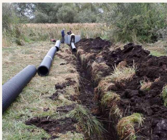
Insertion of sluice to control water levels in Cossington duck decoy, Sedgemoor. Somerset County Council Historic Environment Services provided archaeological supervision whilst the restoration works were undertaken by RSPB volunteers and the landowner (8A1). © Somerset County Council
