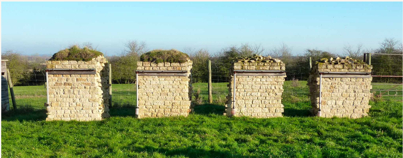
These walls were built for comparing soft and hard caps for protecting walls. They are now to be used for further testing under the Damp Towers research project where the performance of different mortar mixes will be subjected to controlled driving rain and natural drying. This phase of the research is to be undertaken by a PhD student as one of the SEAHA (Science and Engineering in Arts, Heritage and Archaeology) studentships, partly funded by English Heritage with most of the work being carried out at the University of Oxford and University College London. © Historic England, Chris Wood
