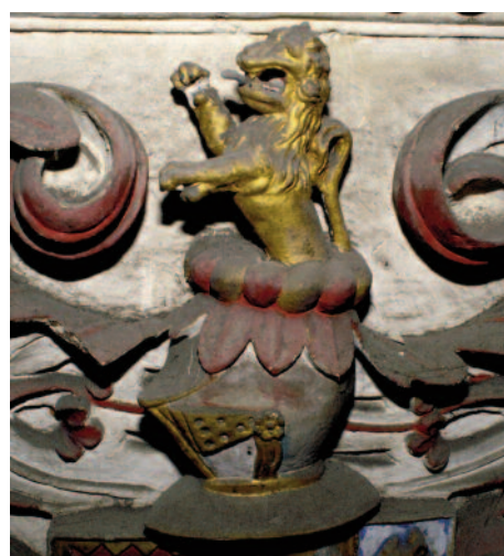
Figure 21 Dust on plasterwork from Chastleton House, Oxfordshire, obscures the original surface finish. Photo: Katy Lithgow
