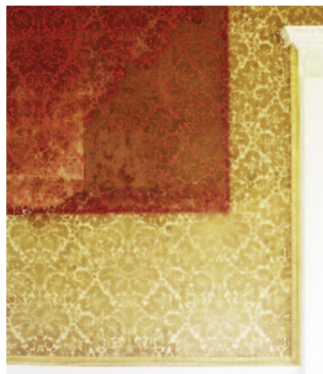
Figure 16 Light damage to the red wallpaper is apparent here in the Red Drawing Room at Uppark House. The red colour has been shielded from the light behind a picture (shown on the right hand side of figure 4). Where the wallpaper has not been covered the red colour has faded to brown. ©NTPL/Andreas von Einsiedel
