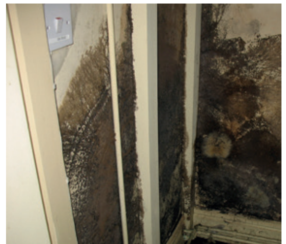
An extreme outbreak of dry rot and mould due to moisture ingress and lack of drying.
