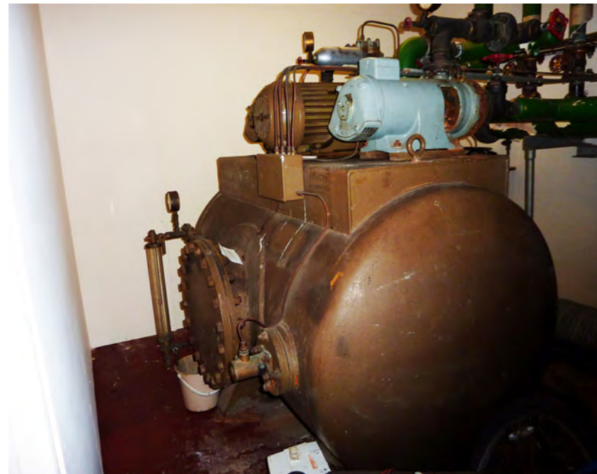
Water booster pump
