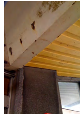
Corrosion in gull wing roof soffit
