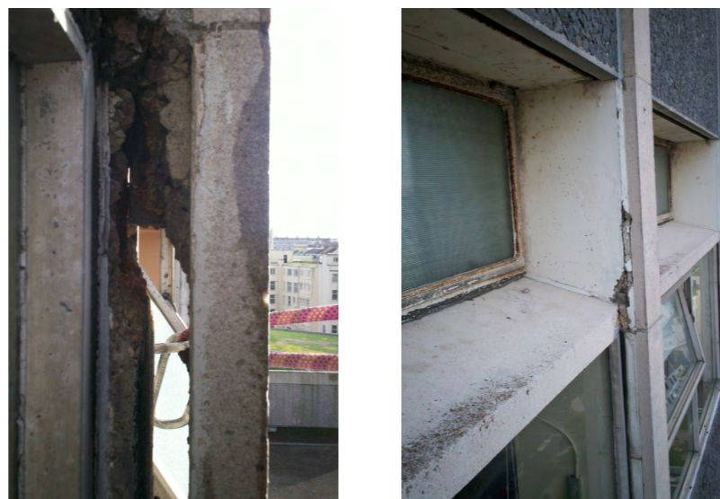
Mortar bed loss and column reinforcement corrosion
