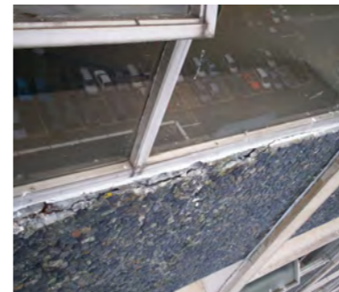
Dilapidated spandrel cladding panels
