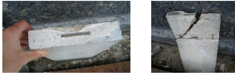
Pilaster cladding panel removed at second floor. Fixing slot visible on left.
